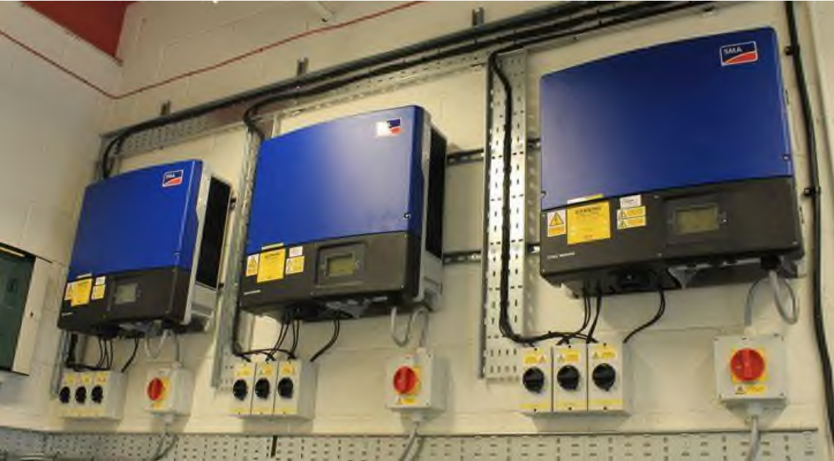
Figure I.1.9 Inverter Representative View Source: https://rudgeenergy.co.uk
