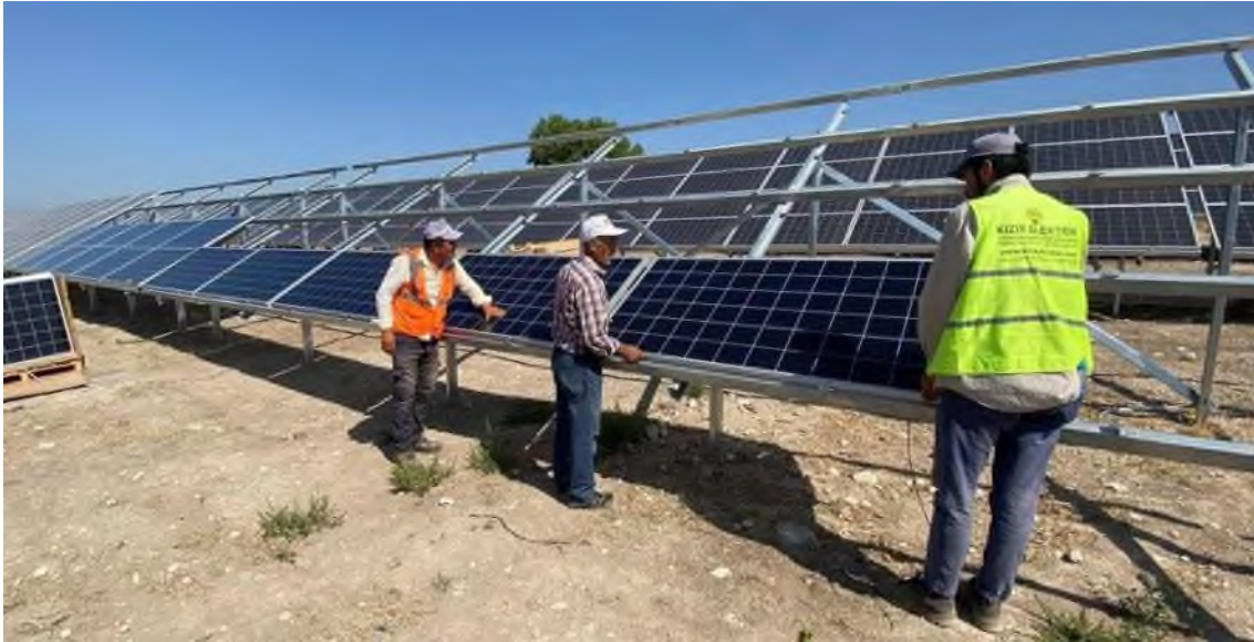
Figure III.1.7.4 Representative Photograph of Placement of Solar Panels on the Carrier System
