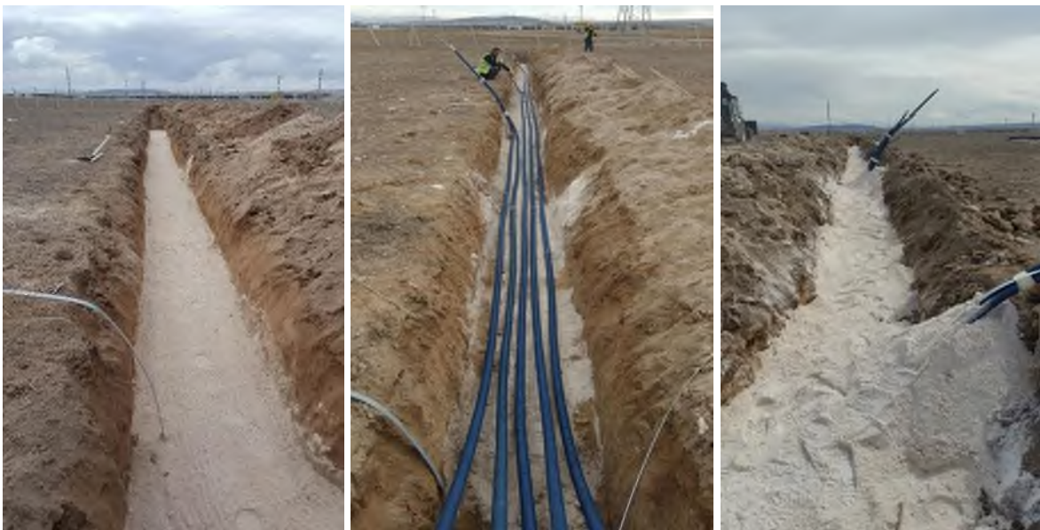
Figure III.1.7.1 Opening of DC and AC Cable Trays Representative Photograph
