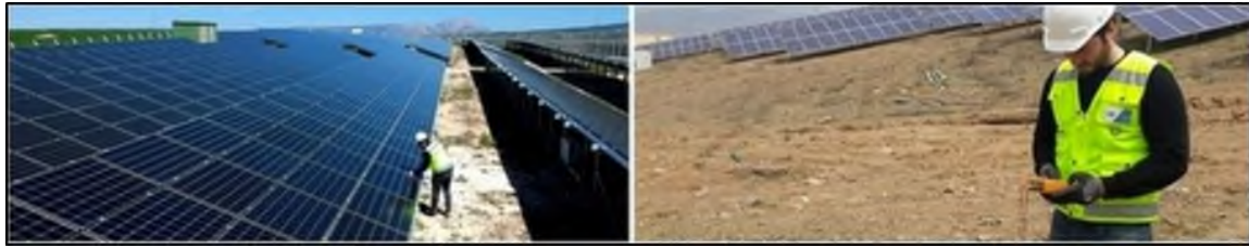
Figure III.1.7.6 Representative Photograph of Test Production and Commissioning of Solar Power Plant
