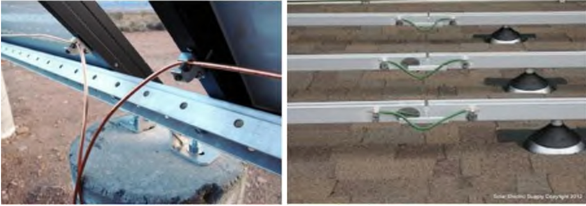
Figure III.1.7.8. Grounding in Solar Panels (Sample View)
